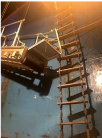
A non-compliant combination arrangement.
